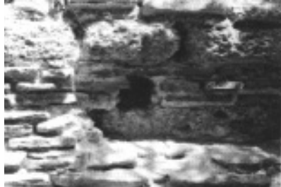
Figure 18. The cavities created due to decaying of wood in “d” section
