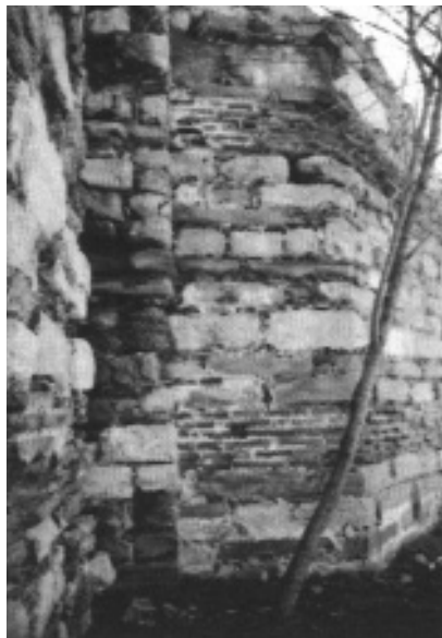
Figure 20. The brick courses end at the corner where walls “e” and “d” of tower II meet
