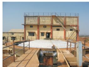
Plate-2 Aeration lagoon at Puikhadee WTP
