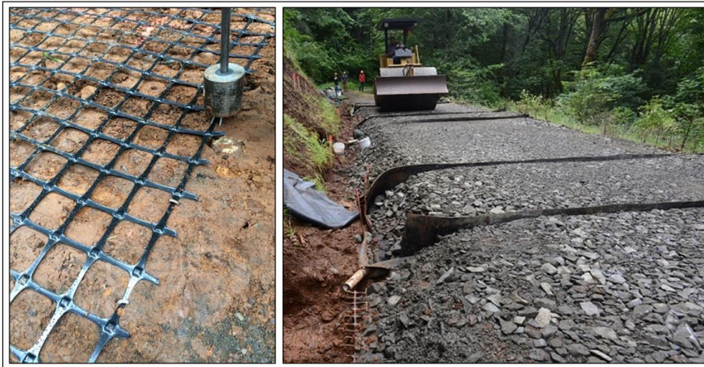
Figure 1. Test track construction: geogrid placement over subgrade (left); buried runoff collection flumes in roadway (right)
