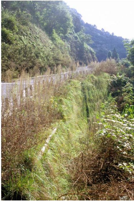
Figure 6. Investigated section where TK wall with vegetation on the surface was prescribed
