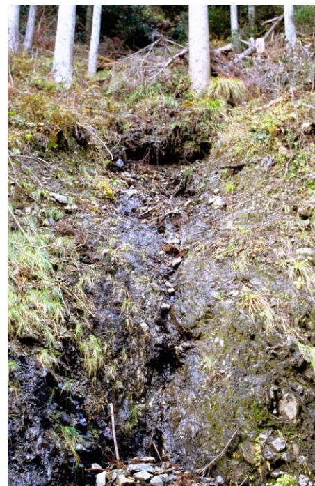
Figure 5. An example of crushing zone and welling water where L-shaped mesh wall was prescribe
