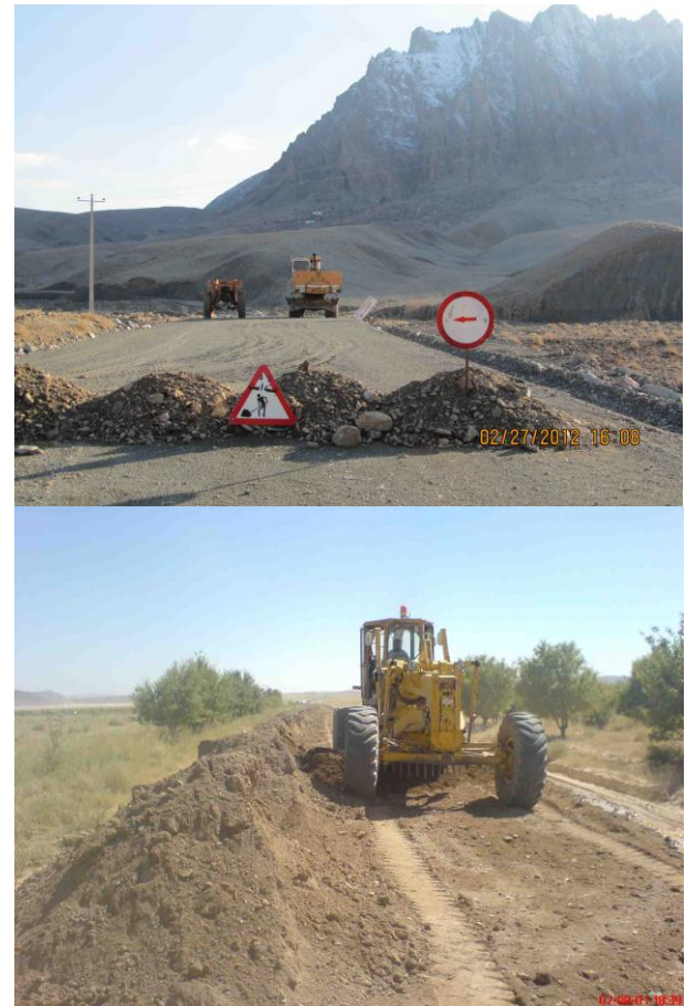
Figures 3 &4. Recently making new infrastructures for rural road in a disadvantaged rural region in semi- arid conditions in South Khorasan Province in -East of Iran (By author, Sep 2010 and Mar 2012).
