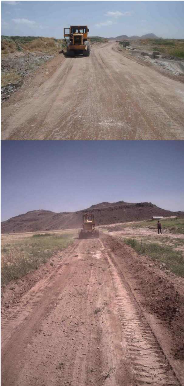
Figures 13 & 14. Establishing and maintaining infrastructures for rural roads in a disadvantaged rural region in semi- arid conditions in South Khorasan Province in -East of Iran (By author, Sep 2010).
