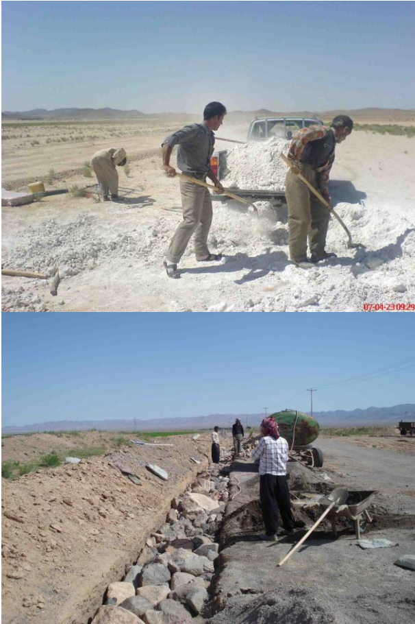
Figures 15 & 16. Using locally materials and workers in establishing and maintaining infrastructures for rural roads in a disadvantaged rural region in South Khorasan Province in -East of Iran (By author, Sep 2010).
