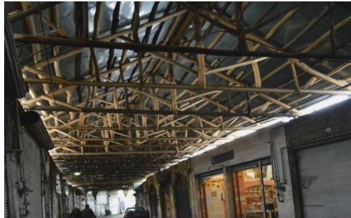
Figure 16. Marketplace's roof before the restoration (source: cultural heritage)
