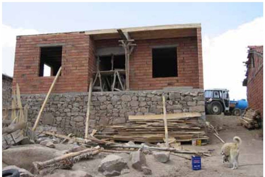
Figure 6. This house in construction exhibits a mixture of newer mass-produced terra cotta brick with little reinforcing constructed on a base of new quarried stone. The work is being done by the family and a hired usta (A. Snyder, 2002).
