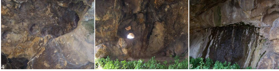
Image 4. One of the shafts on the ceiling. Turbulence holes are visible on the left.
